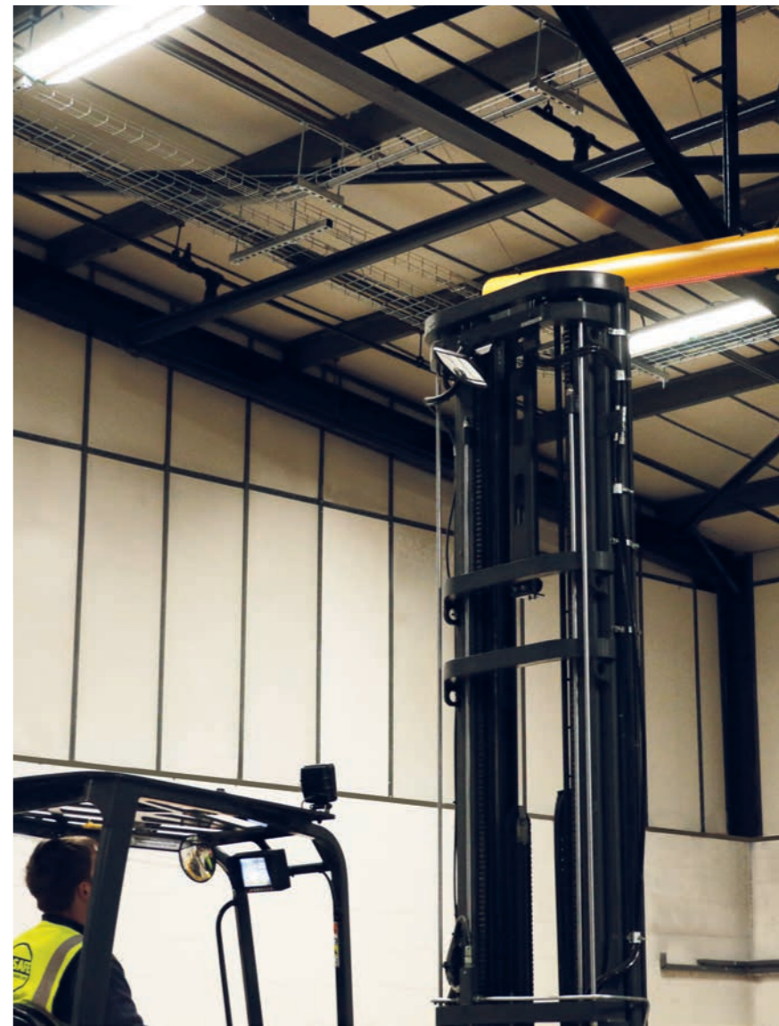
Protect low hanging infrastructure in environments where high-level vehicles such as forklift trucks are in operation.
